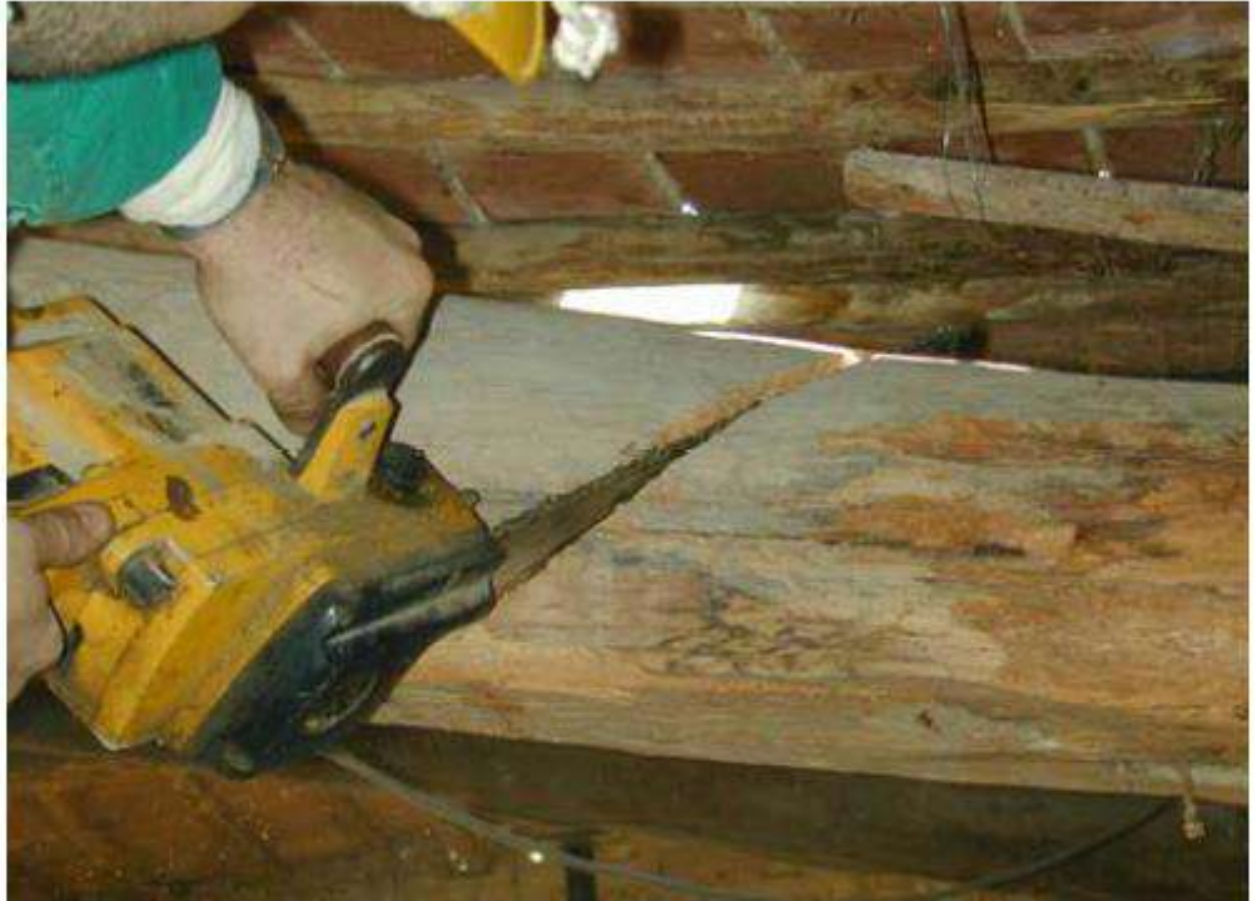
Inclined cut of decayed end
