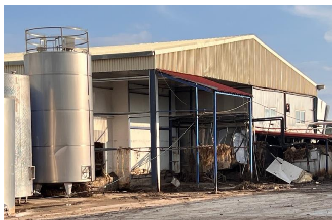
Figure 15: Completely destroyed Feta cheese factory.
