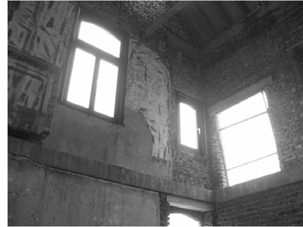
The existing slabs and division walls were removed, leaving the shell of two-and-a-half floors empty.
