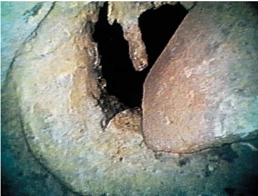
PLATE 4. Video probe image of interior of joint in Fig. 47. Metallurgical joint in the Jockey's neck. Excess flow weld metal visible in center. The shard on the right is lodged in throat. Photo by the author.
