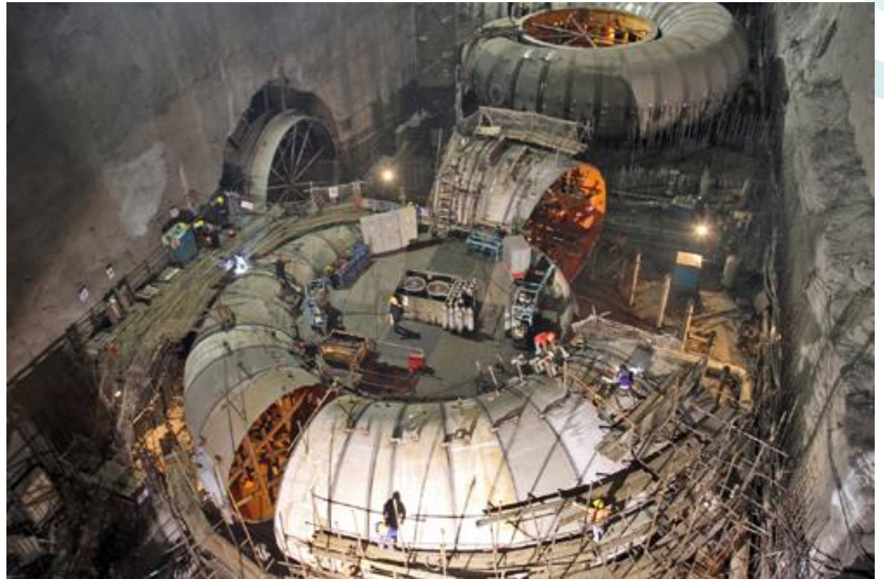
14 MW. Xiluodu Hydropower Station, China
