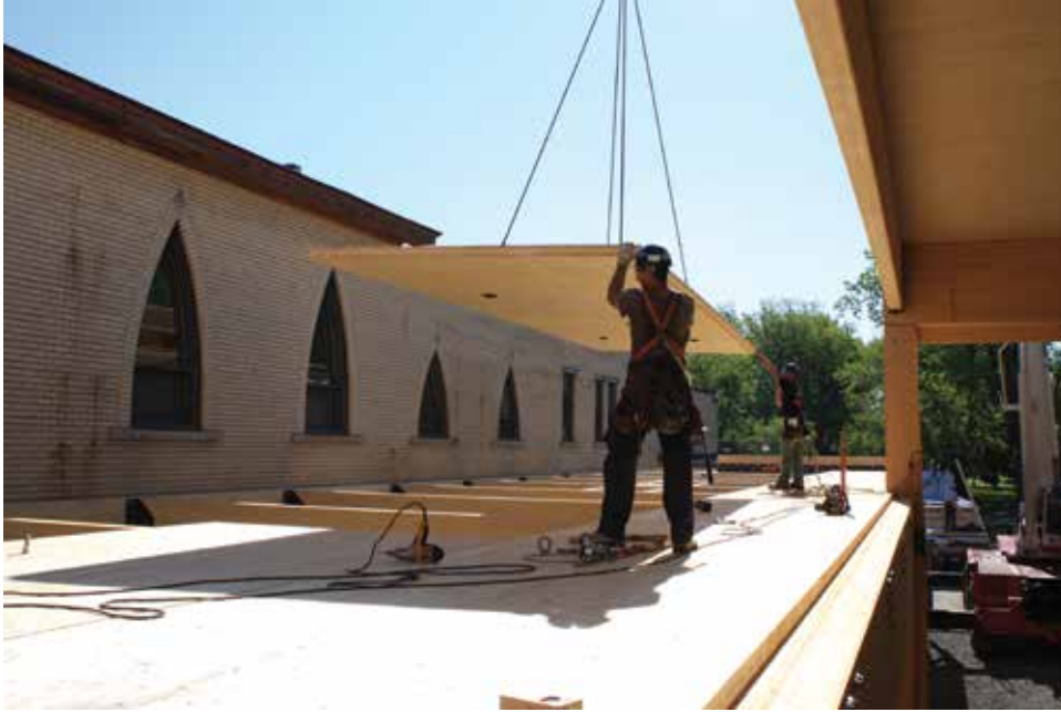
Figure 8 Lifting and handling of CLT elements, in Canada (courtesy of Nordic Engineered Wood)
