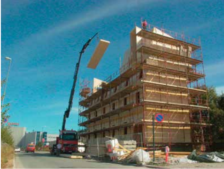
Figure 10 Lifting and handling of CLT elements, in Norway (courtesy of Brendeland and Kristoffersen Architects)
