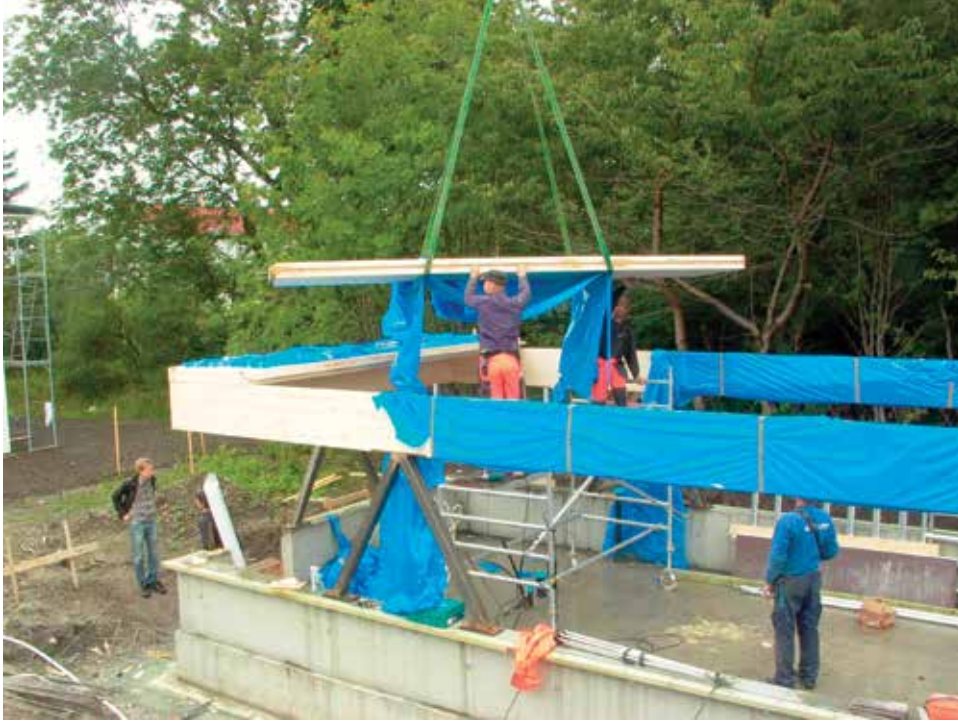
Figure 4 Lifting and handling of relatively light CLT elements, in Norway (courtesy of Brendeland and Kristoffersen, Architects)
