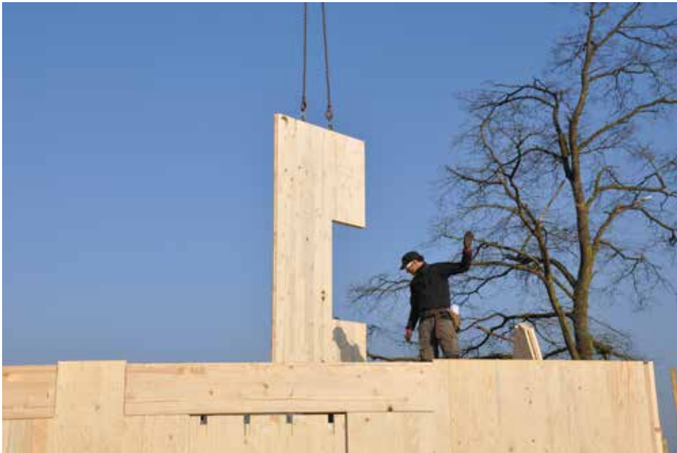
Figure 5 Lifting and handling of CLT wall elements, in Belgium (courtesy of HMS)
