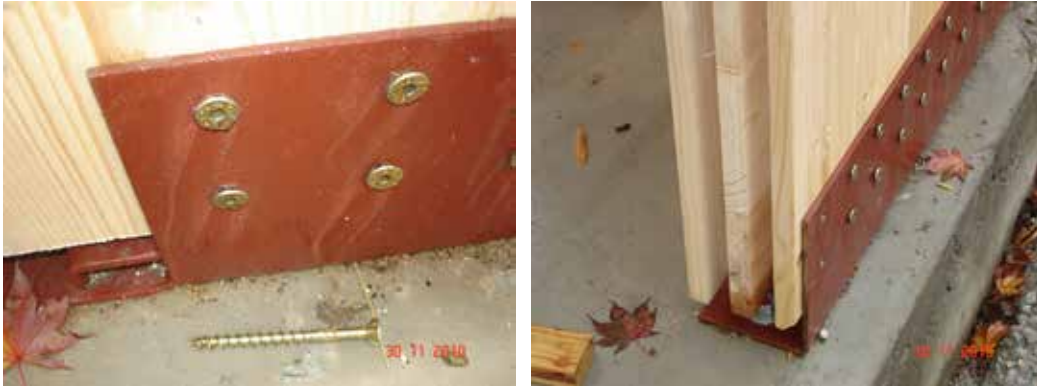
Figure 30 Example of a connection detail with a gap between CLT wall and concrete foundation
